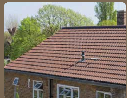
Landmark Double Roman, Brown Brindle, Hackney Homes, Hill Court Estate, Hackney, London
